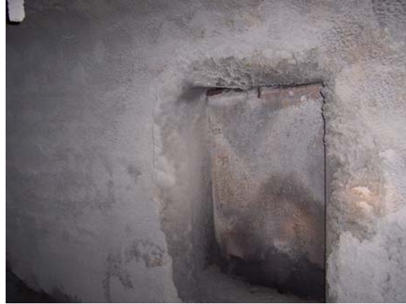
Concrete Block Stopping in Poor Condition.
