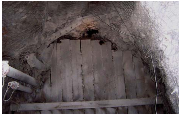
Kennedy Stopping in Poor Condition.
